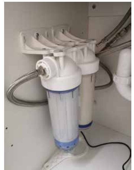
FIG1: OSMIO EZFITPRO-300 INSTALLED WITH HOSES. IT IS AN EASY WAY TO DO IT IN SOME CASES AND YOU CAN BUY THE HOSES FROM ANY PLUMBERS MERCHANT
